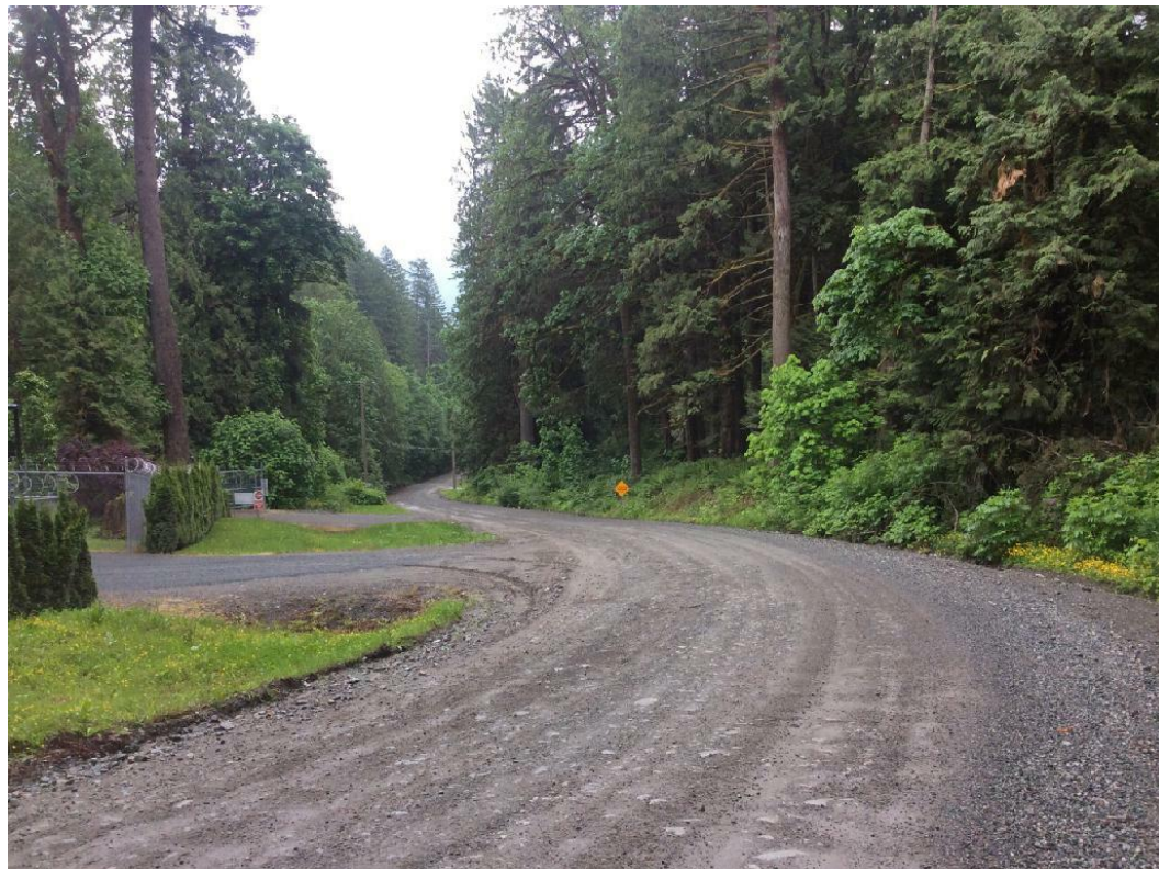
Photo 4 1.5 km Chehalis FSR, road section with washboard surface
