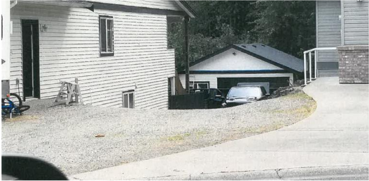
Image of the constructed shop from Berston Road (August 12, 2020). Covenant BT217825 requires floor area to be 0.4 metres above Berston Road. The shop does not meet this requirement
