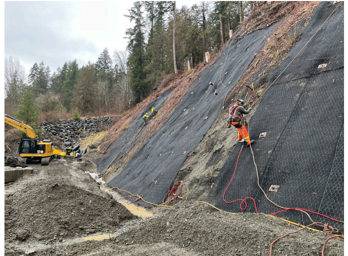
Workers install 950m 2 of geomattening and 24 soil anchors via high-angle rope work, at the Guy Creek Debris Basin engineered slope in the Chilliwack River Valley, Area E.
