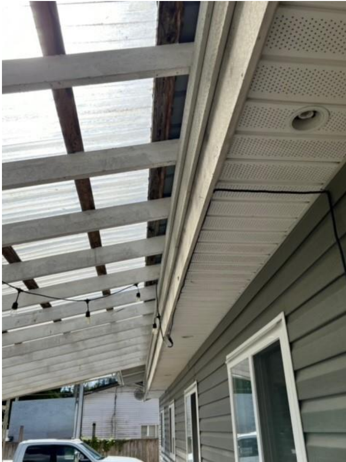
Figure 2: The rear deck cover was attached to the roof of the dwelling to act as one continuous structure. A building permit will address this connection to the dwelling if the BOV application is successful.
