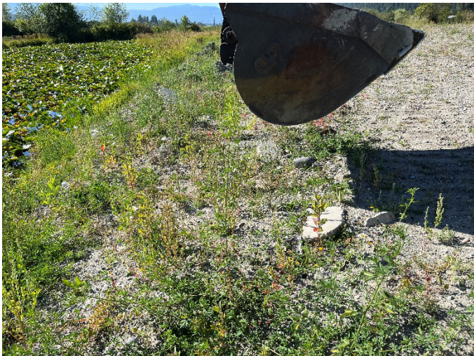
Figure 11. Photo showing some pieces of concrete in the fill material that had been imported.
